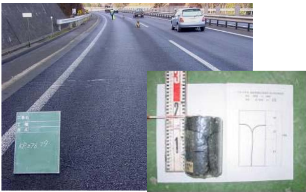
Picture1 Damage under porous asphalt
