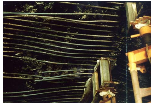
Figure 4.1 Serious damage of concrete slab by fire
