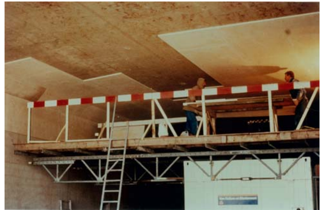
Figure 5.3 Fire protection panel are fixed on the concrete surface (photo by RWS, Netherlands)
