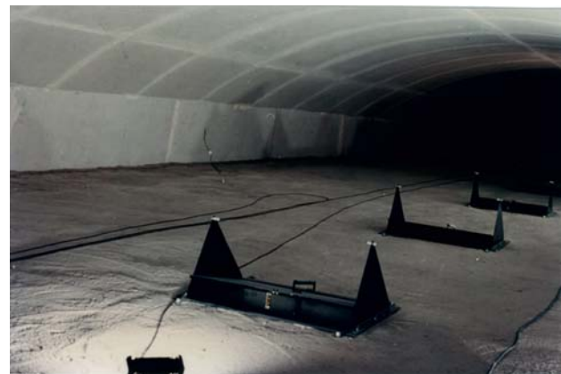
Figure 5.4 Fire protection panel are fixed on the circular ceiling (photo by 4th Elbe Tunnel, Germany)
