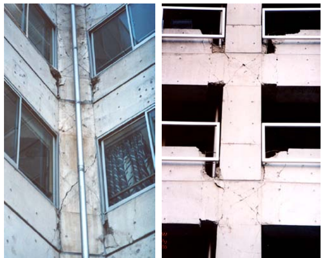
(b) Shear failure and damage of columns
