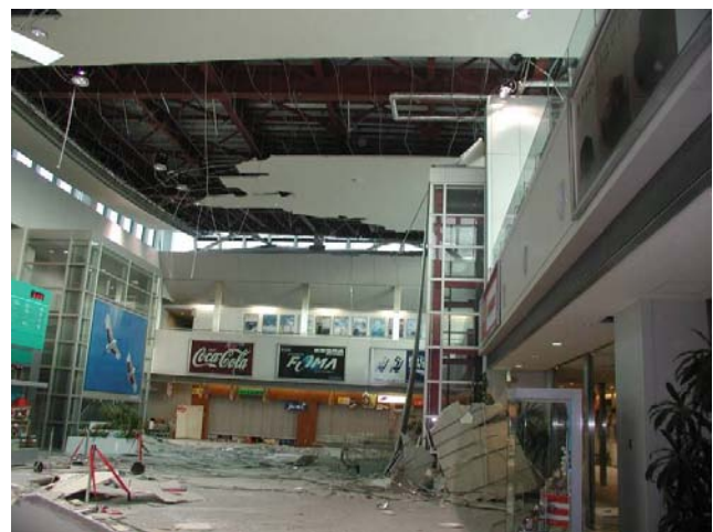
Figure 2 Ceiling of the airport terminal fell down by the Off Tokachi Earthquake in 2003
