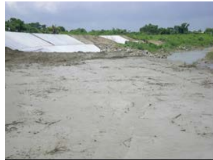
Picture 1 A broken embankment next to a nursing home in Taiwan
