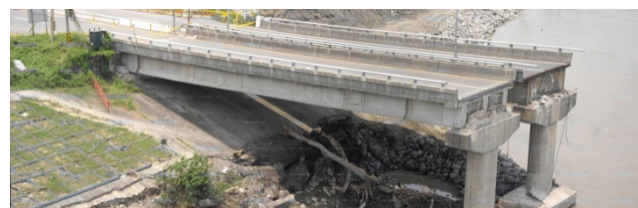
Figure 3 Shuang-Yuan Bridge failed in scoring photoed by AUMAV
