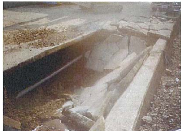
Fig.1 Breaking situation of pipeline
