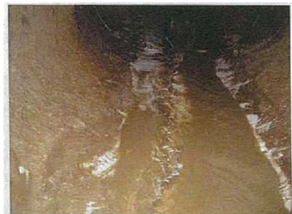
Fig.2 Inner situation of deformed pipe
