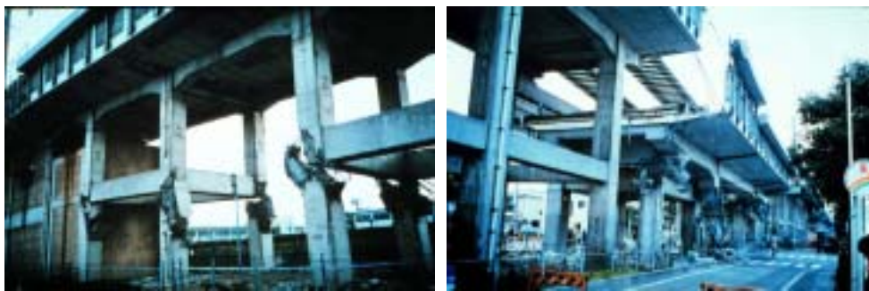
b) Shear failure of railway viaduct
