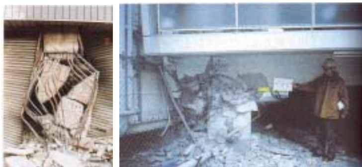
d) Shear failure and collapse of first floor building column
