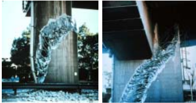
a) Shear failure of highway bridge pier
