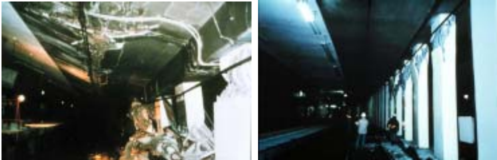
c) Shear failure of intermediate column leading to collapse of underground subway
