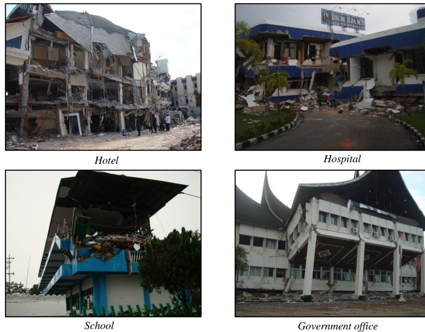
Figure 3.6 Critical Facilities Damages due to September 30, 2009 tsunamigenic earthquake (Source: H.P. Rahayu Photo 2009)
