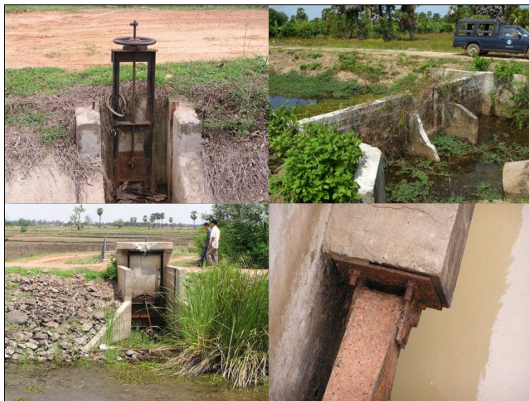
Figure 2 Examples of malfunction small-scaled water resources project
