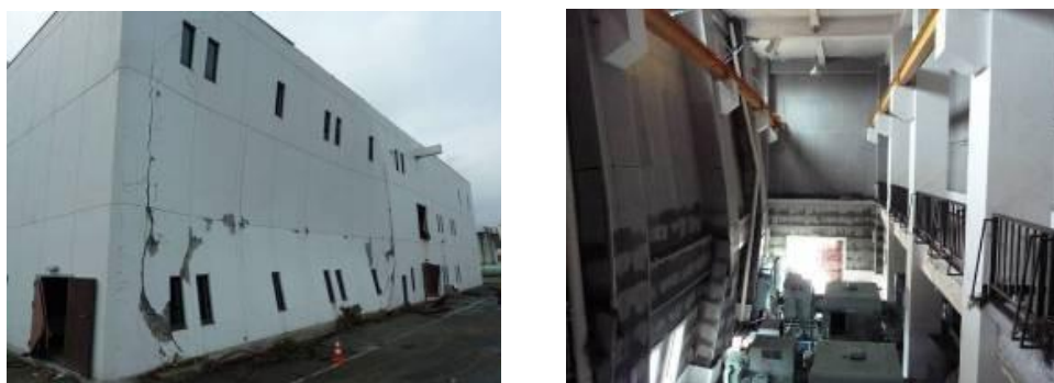
Fig. 1.14 Three-story RC wall-frame building damaged by tsunami [57]
