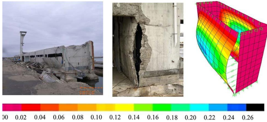
Fig. 1.16 FEM analysis of a large fish market building damaged by tsunami [56]
