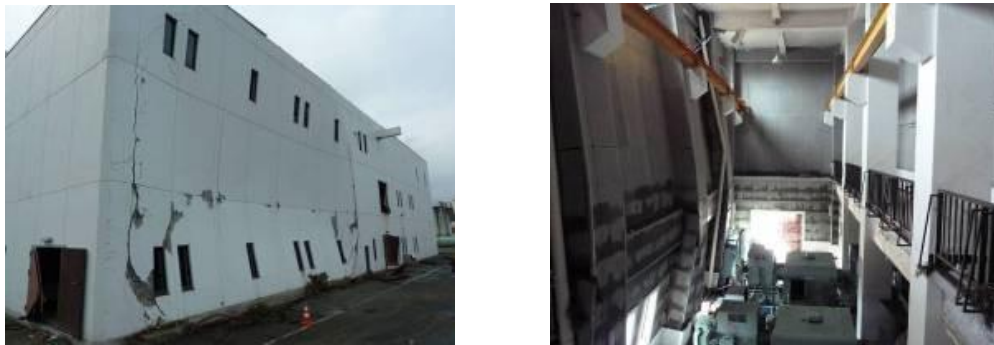
Fig. 2.14 Damage of a three-story RC wall-frame building [57]
