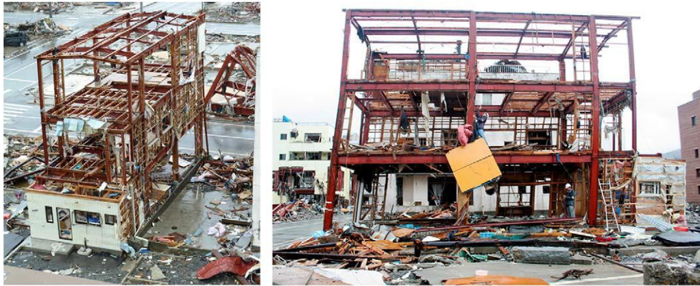
Fig. 1.15 A three-story steel-frame building damaged by tsunami [56]
