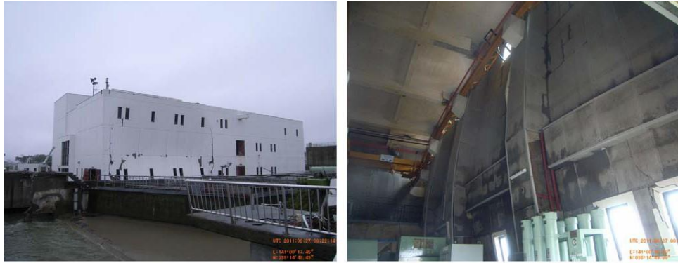
Fig. 1.18 Ocean-facing RC wall damaged by direct strike from tsunami bore [56]
