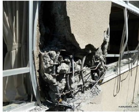
(b) Damage of column [2]
