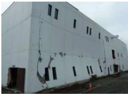
(c) Damage of RC wall [4]
