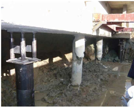
(a) Damage of pile head [3]
