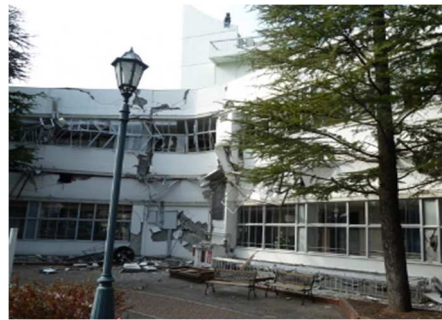
(d) Damage of RC building [2]
