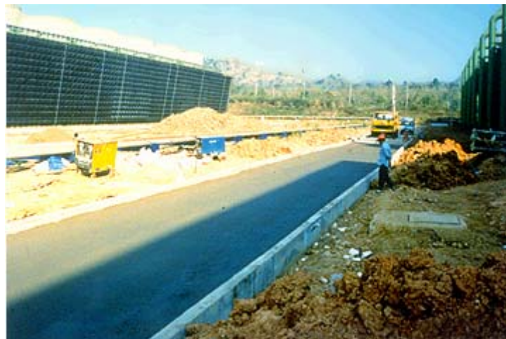
Fig.6 Demonstration construction of Roller-Compacted Concrete Pavement using fly ash at Mae Moh power generating plant
