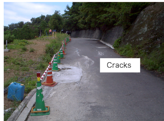
(a) Cracks on the road
