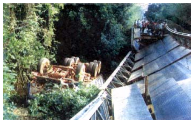
Fig.2 the collapse of a bridge on the road from Siem Reap to Bantey Srey temple on April 10, 2004
