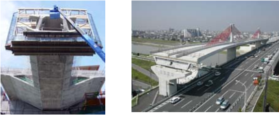
Fig.19 “Fragmental” construction in city center, Shin-Meisei bridge, (Nagoya city expressway and Sumitomo)
