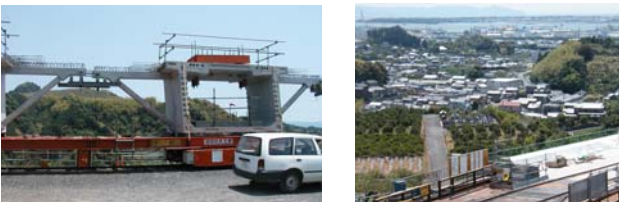
Fig.21 Struted top slab, in suburban farming areas, Yamagiri viaduct, (JH and Sumitomo)
