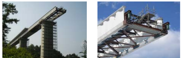
Fig.24 End span using UHPC serving as erection nose during launching, Torisaki-gawa bridge, (JH and Taisei)
