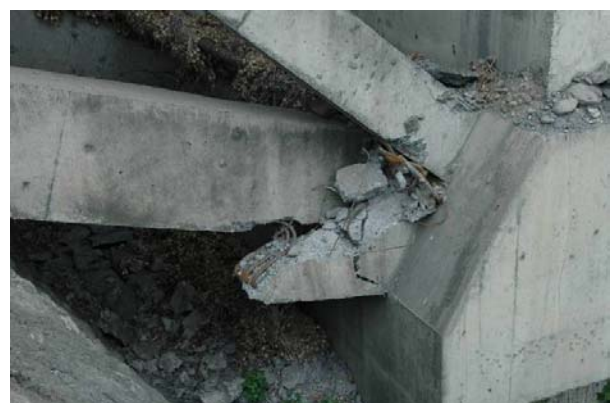
Fig. 27 The fractured element of Xiaoyudong bridge
