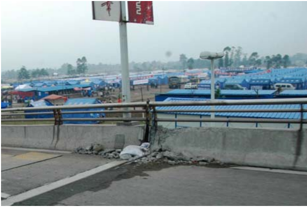
Fig. 32 The damaged expansion joint
