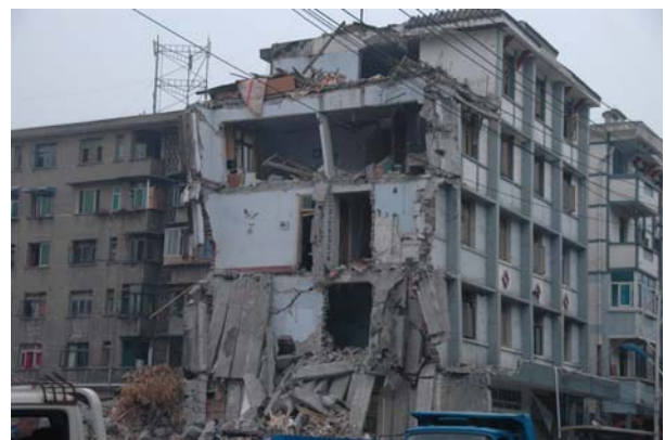
Fig. 5 The collapsed residential buildings (URM)
