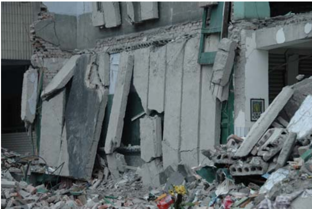
Fig. 1 The close-up view of the collapsed classroom
