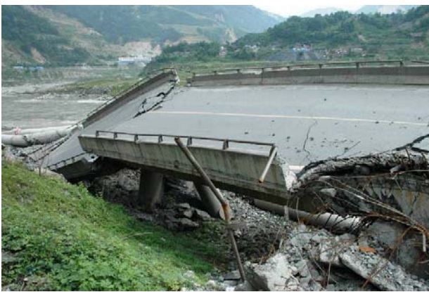
Fig. 23 The collapsed decks of Baihwa bridge
