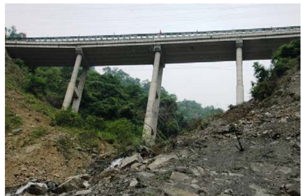
Fig. 30 The damaged bridge in Highway 213
