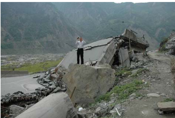
Fig. 24 The collapsed Baihwa bridge
