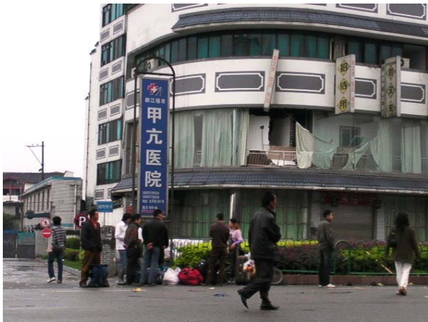
Fig. 13 The structural damages of a hospital
