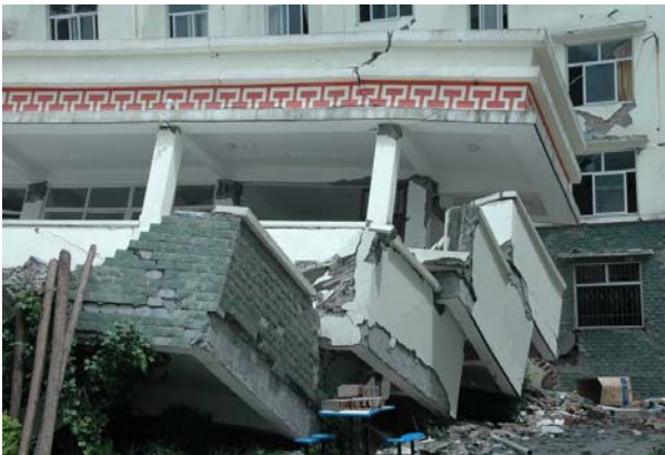
Fig. 7 The collapsed RC school building
