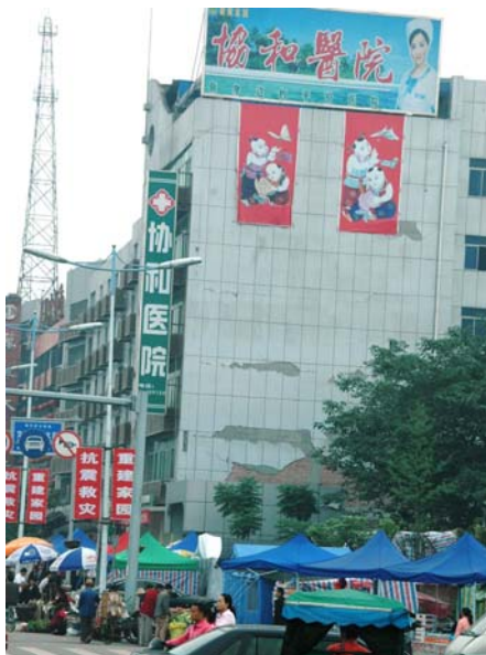
Fig. 12 The hospital suffered medium damages
