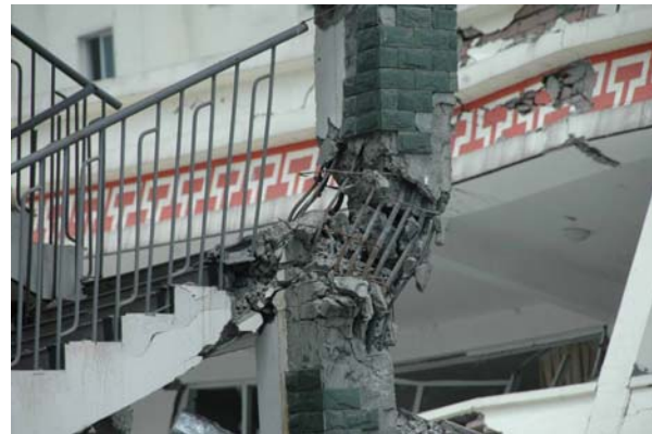
Fig. 10 The close-up of a damaged RC column
