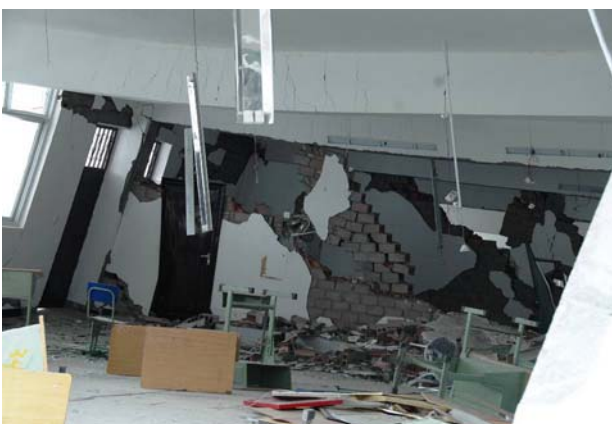
Fig. 8 The damaged classroom
