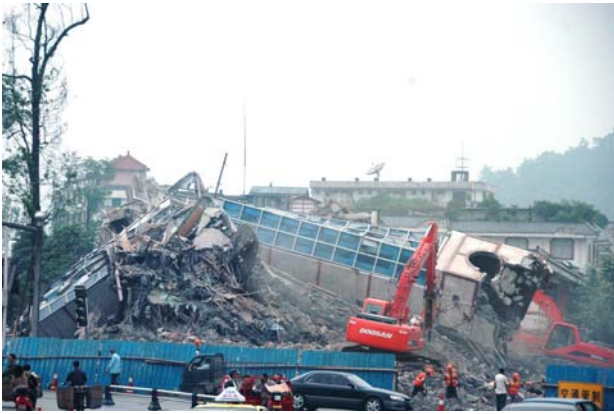
Fig. 6 The collapsed commercial buildings
