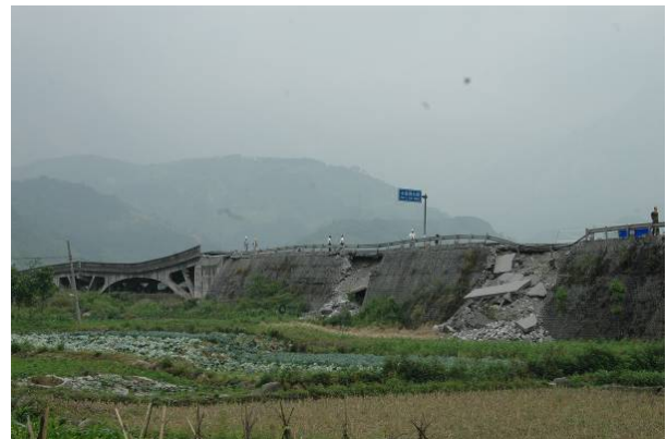
Fig. 26 Fault rupture went through the embankment of Xiaoyudong bridge
