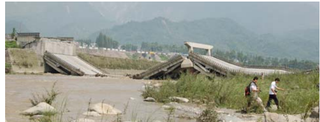
Fig. 25 The collapsed spans of Xiaoyudong bridge
