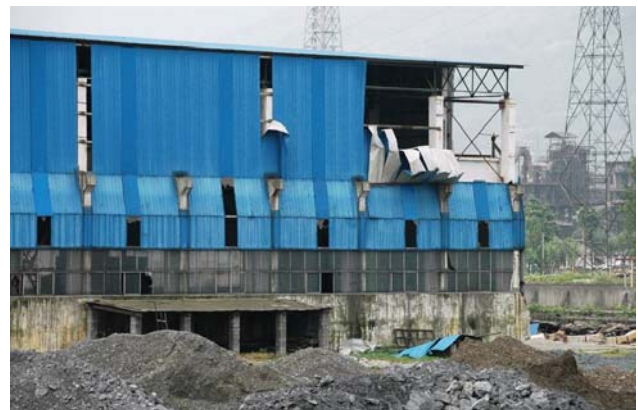
Fig. 15 The damaged factory
