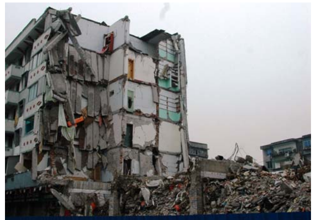
Fig. 4 The collapsed residential buildings (URM)
