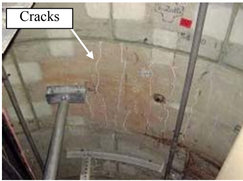
Figure 9 Cracks on the segments
