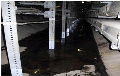
Figure 10 Inflow of groundwater into the tunnel
