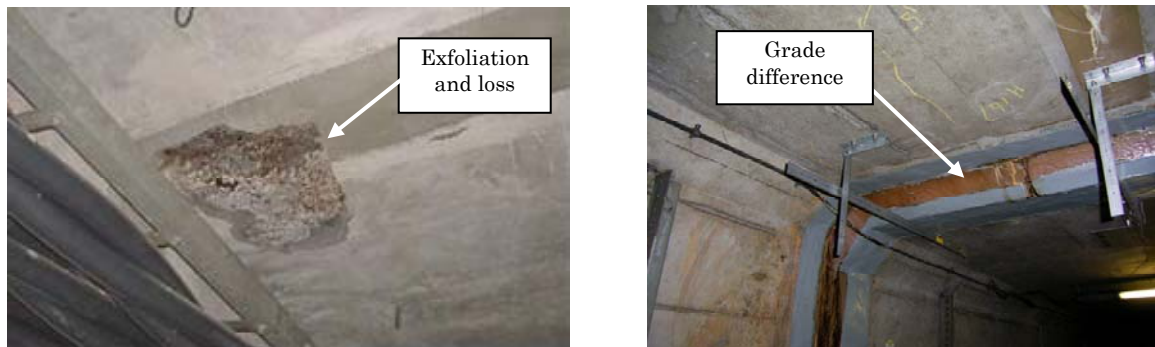
Figure 4 Example of tunnel at abnormal state
